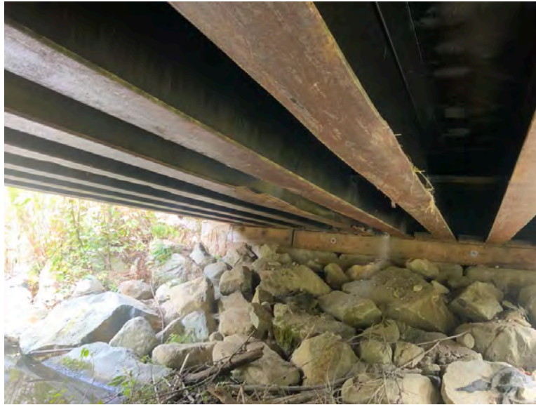
Stringers, dents likely done during installation
